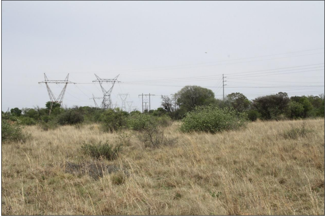
Figure 8: Power lines near the Watershed Substation.
