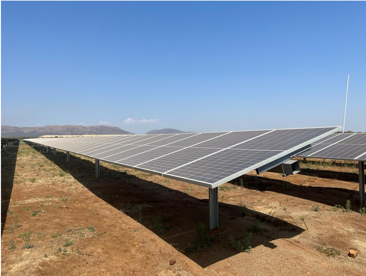
Figure 1-2 A Typical Photovoltaic Solar Energy Facility
