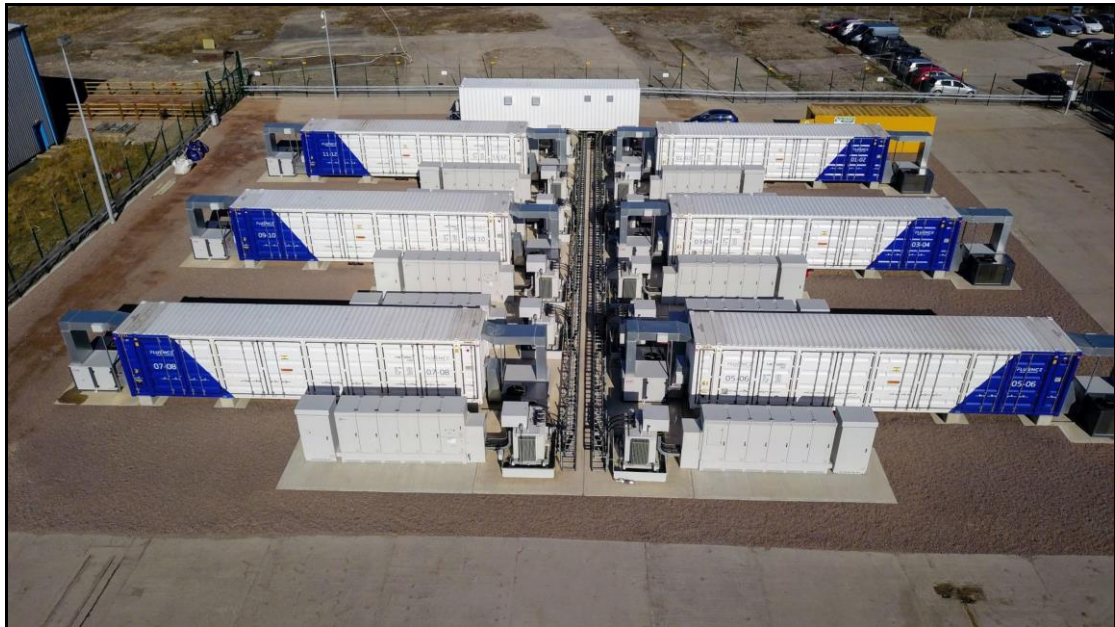
Figure 3: Aerial view of a BESS facility (Photo: Power Engineering International).
