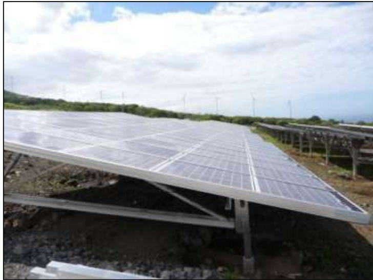
Figure 11: Fixed Solar PV Panels
