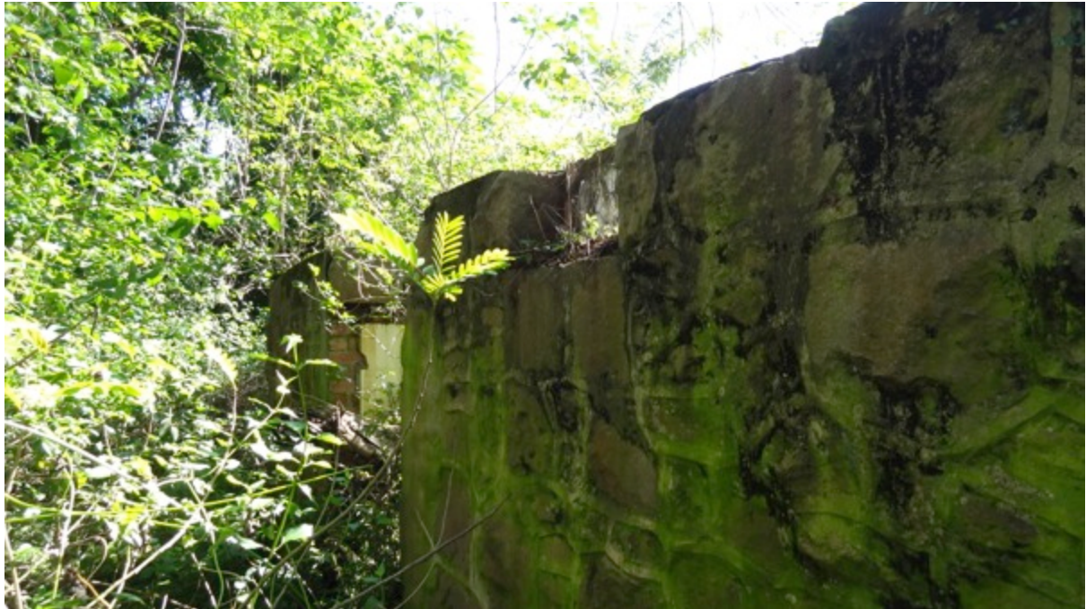
Figure 12: Plate 11: View of derelict stable as seen during the site condition survey in May 2013 This structure has been renovated several times in its history of use(Photo: Author, May 2013).
