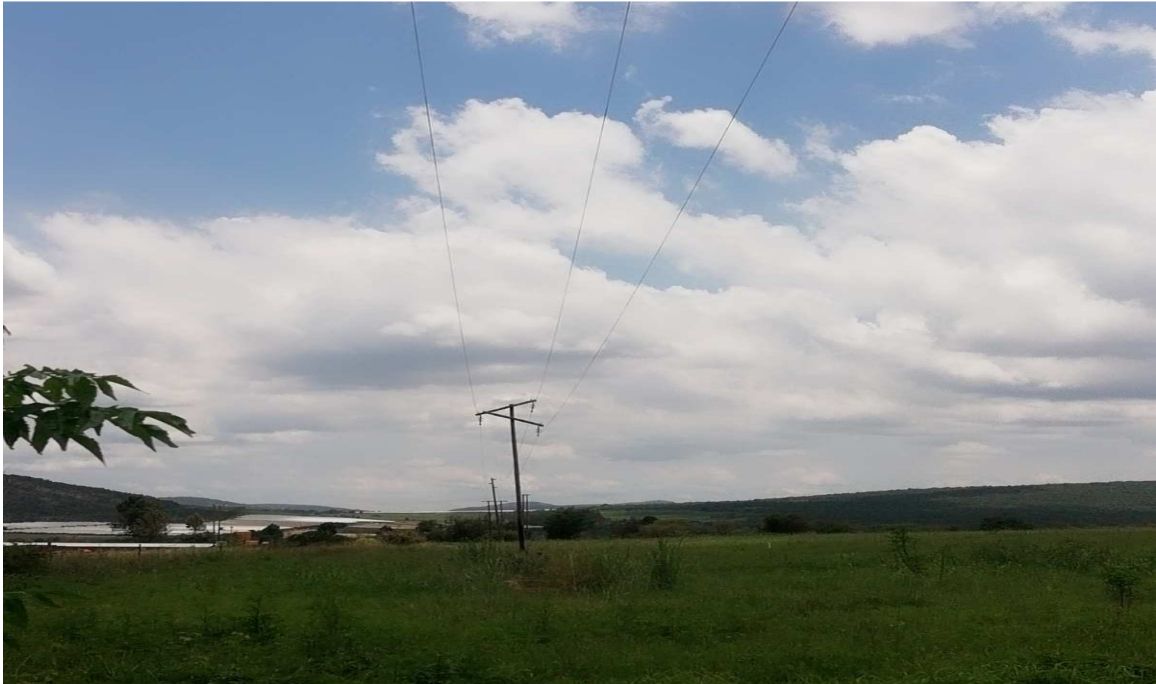
Figure 3: Existing electrical infrastructure
