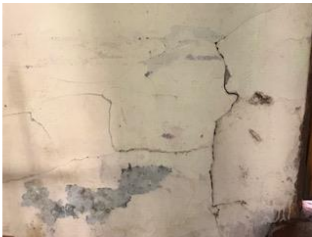
Figure 4: Damage to brickwork Ludeke Methodist Church
