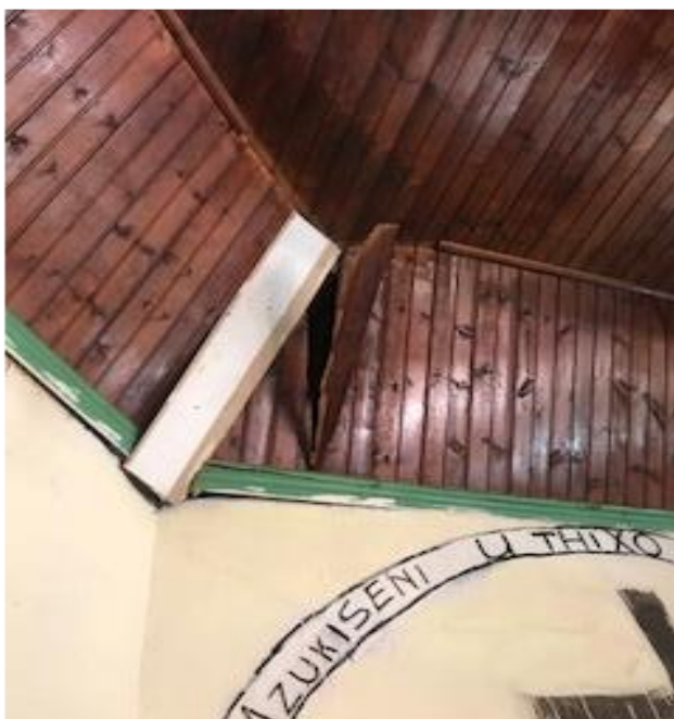
Figure 2: Opening on the roof of Ludeke Methodist Church in Mbizana Eastern Cape
