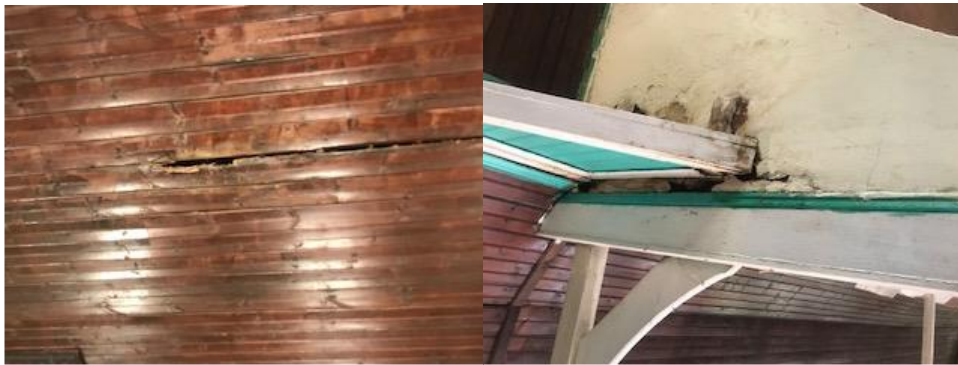
Figure 3: Fascia Boards rotting of Ludeke Methodist Church in Mbizana Eastern Cape
