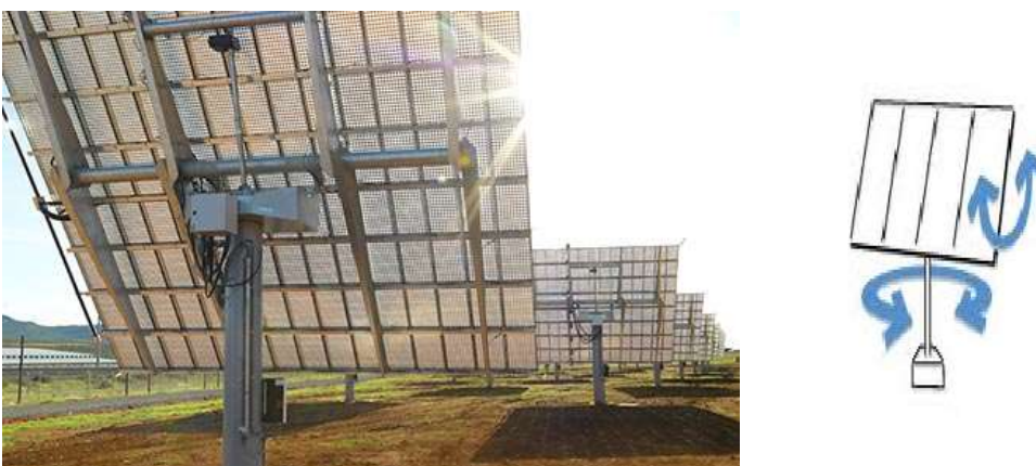
Figure 12: Examples of double axis PV tracking systems (Solek, 2016)
