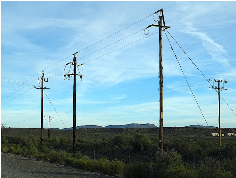
Example of the existing 22kV Eskom powerline and adjacent telephone line
