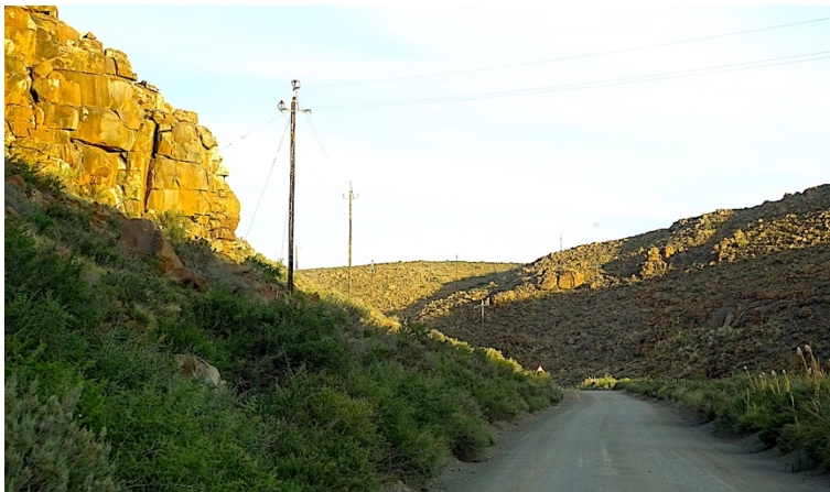
The 22kV Eskom powerline crosses the R381 Route twice over a short distance in the scenic Sakrivier poort.
