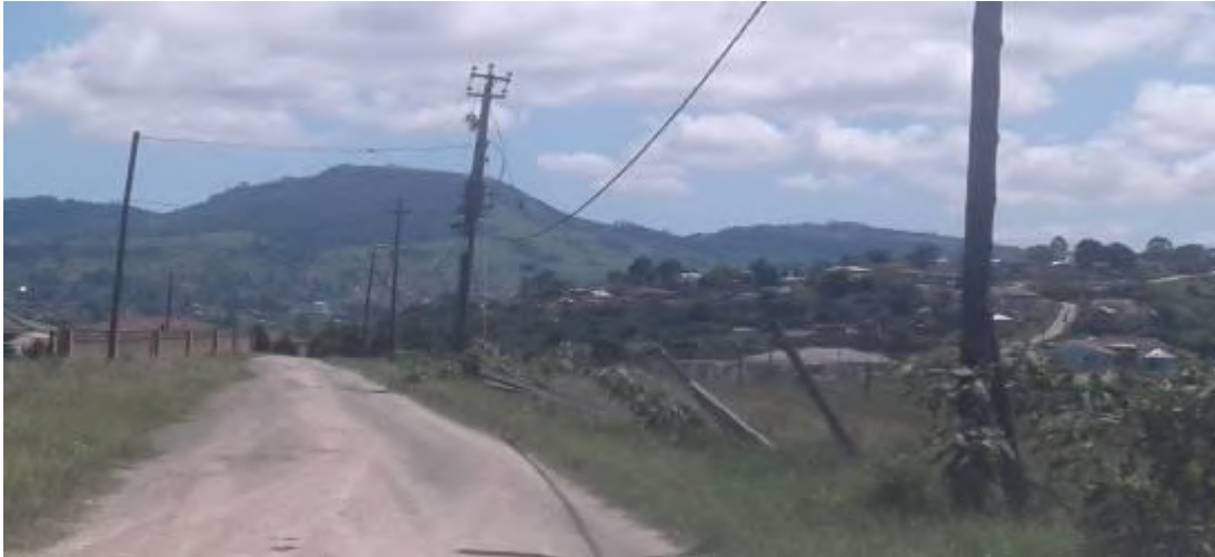
Figure 8: Existing Eskom network feeding the existing houses
