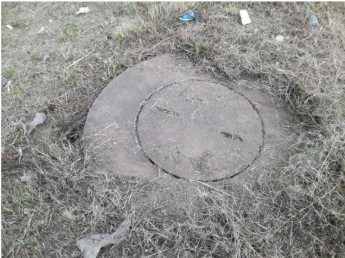
Figure 5: Existing sewer reticulation on-site feeding the existing houses
