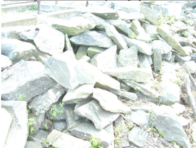
(b) The rough stone walls are falling apart as a result of weak foundation.
