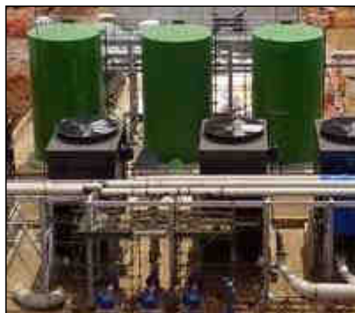
Plate 2.19: Liquor storage tanks.
