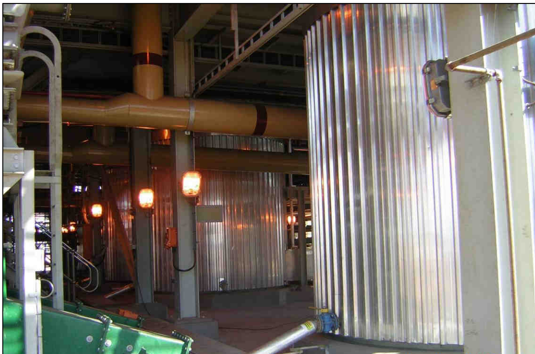
Plate 2.16: Tar storage tanks.
