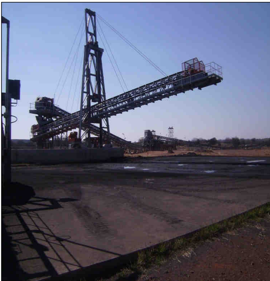
Plate 2.6: The coal from the mine is transported to the Char Manufacturing Plant Expansion via conveyor and is stockpiled on a concrete lined area.
