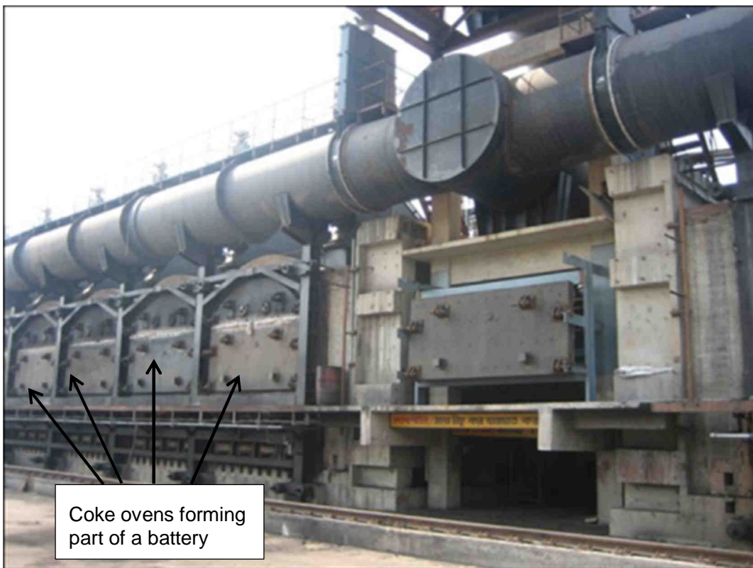
Figure 2.3: Part of a coke oven battery (similar to proposed Market Coke Plant).
