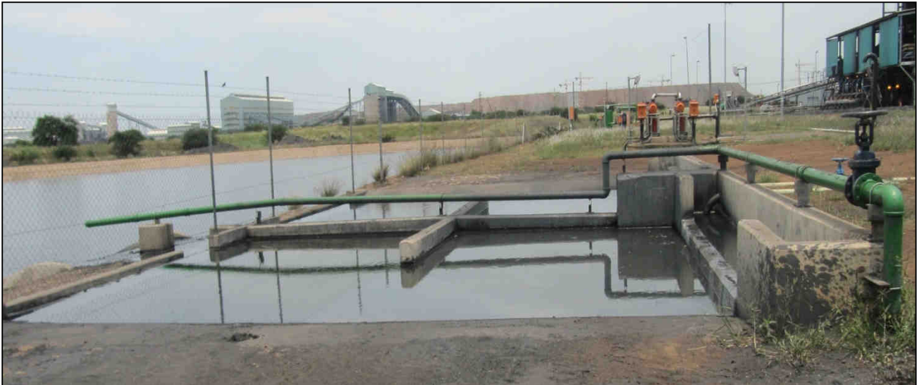
Figure 6.3: Existing silt trap to remove silt before water enters the PCD and PCD extension.
