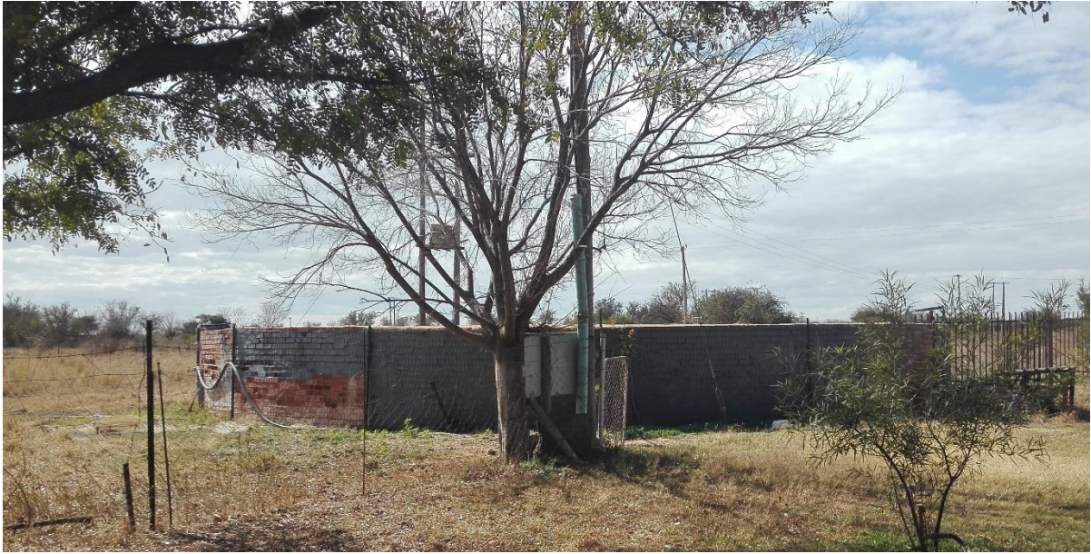
Photograph of the site, showing the reservoir to catch rain water
