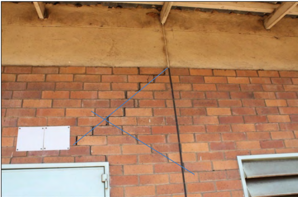
Figure 8: Example of blast induced damage.
