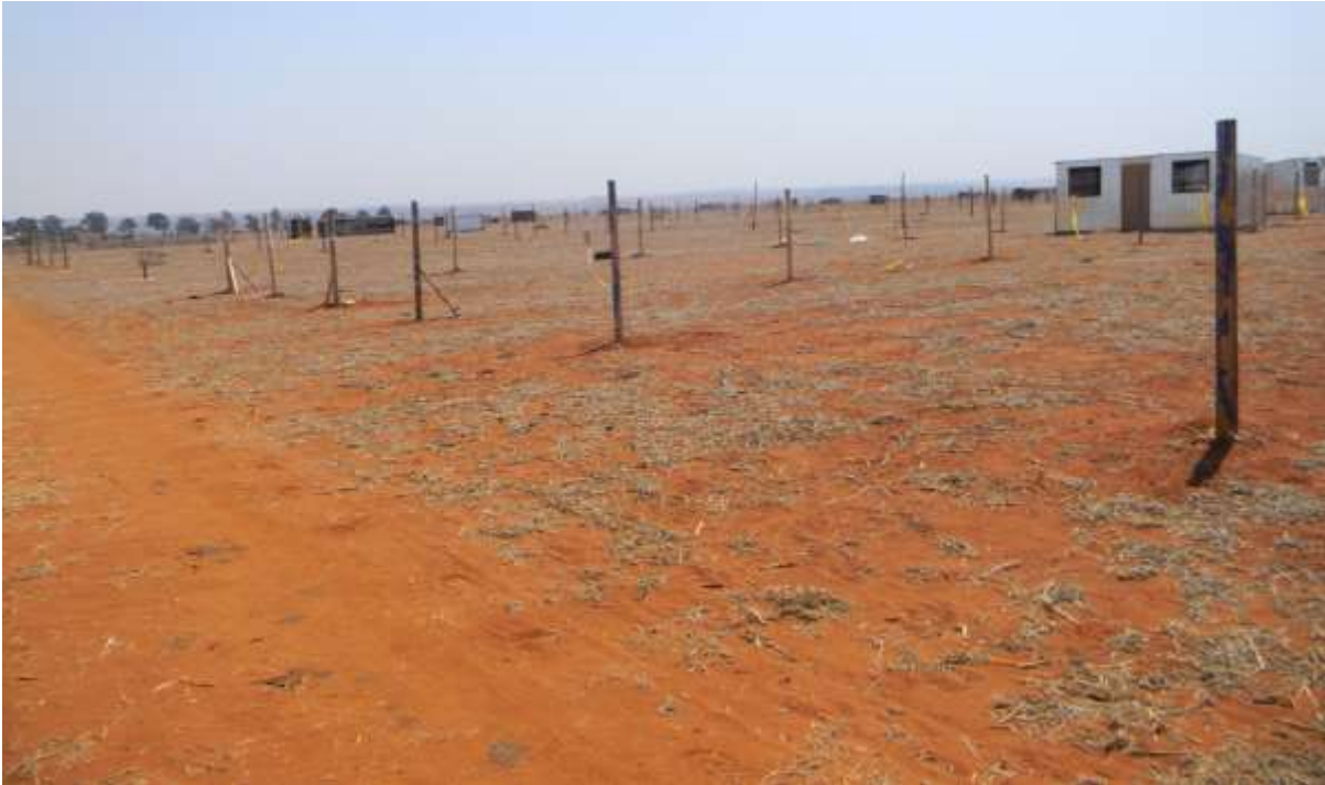
Plates 6: Shows new houses being erected at the site earmarked for township establishment.
