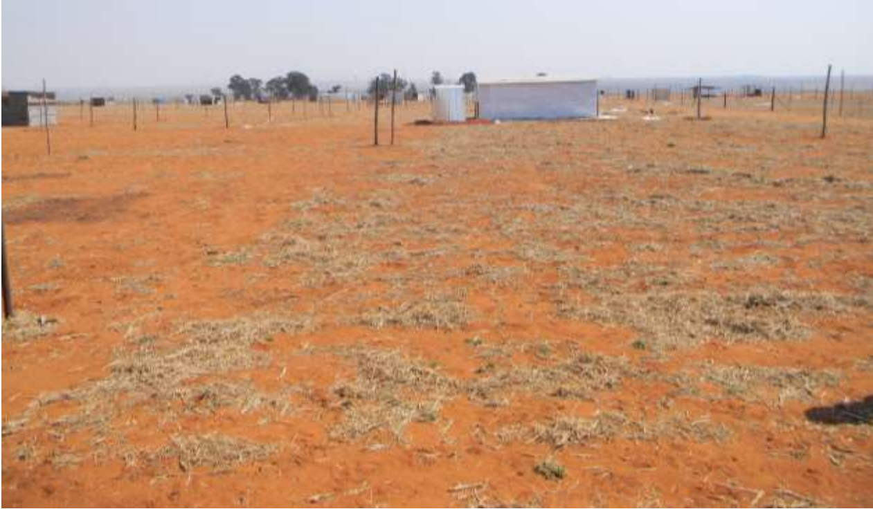
Plate 9: Shows new informal houses being built at the site earmarked for township establishment by Mpumalanga Department of Human Settlement.
