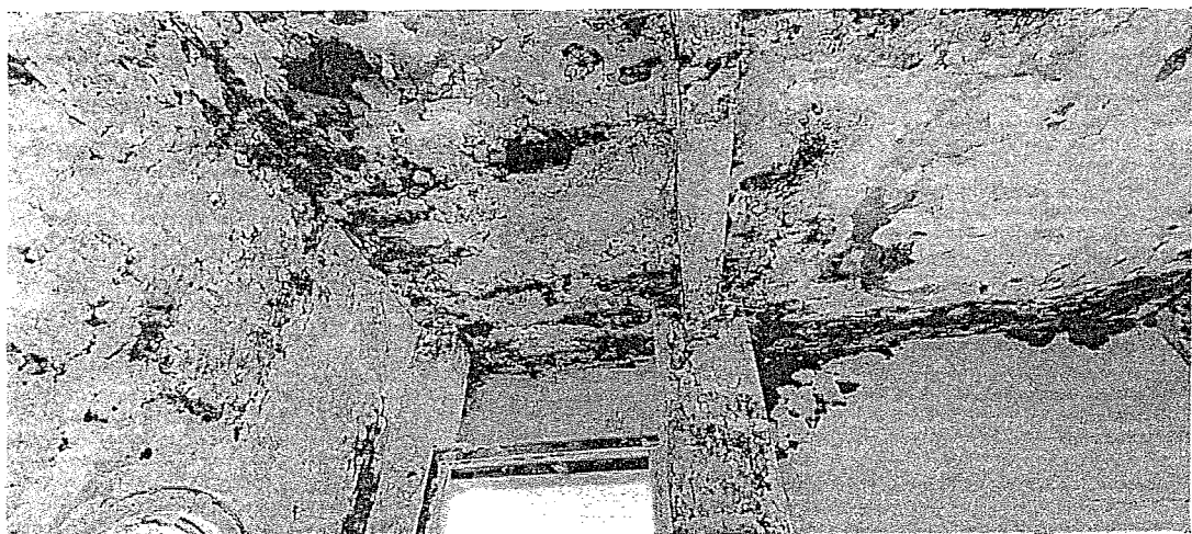
SLIDE 3 : SPALLING ALONG SOFFITS AND MOISTURE INDUCED DAMAGE
