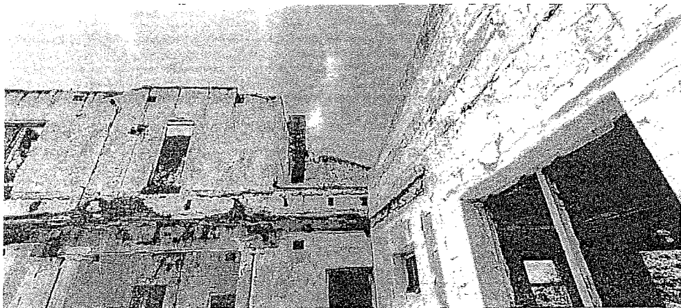
SLIDE 1 : MOISTURE INTRUSION ALONG EXTERNAL ENVELOPE
