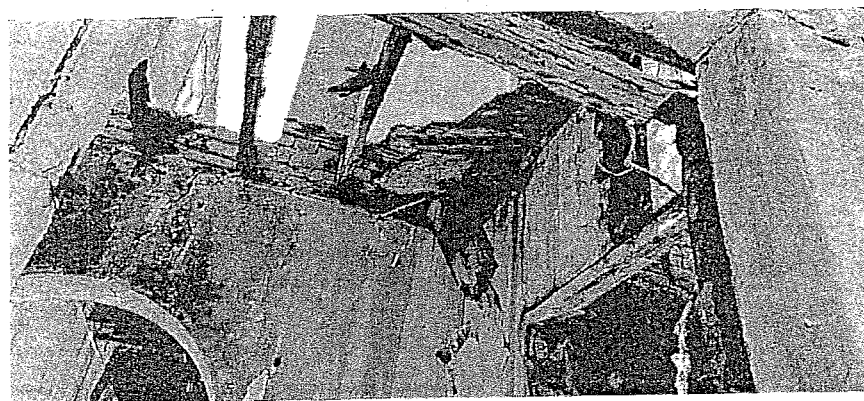
SLIDE 7 : DAMAGED TO ROOF AND INTERNAL ENVELOPE
