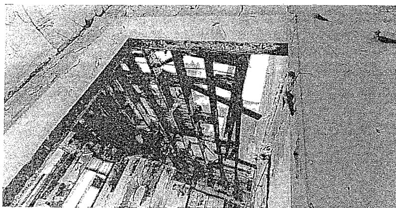
SLIDE 8 & 9 : DAMAGES TO ROOF
