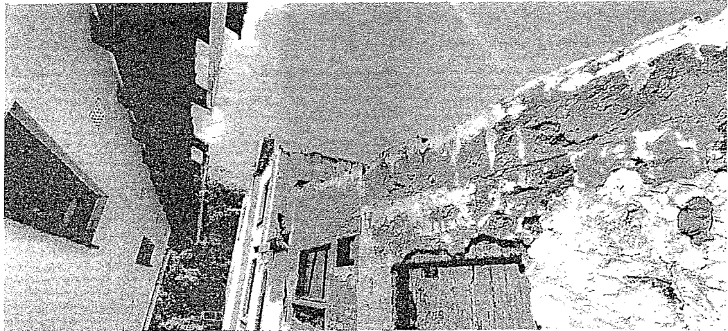
SLIDE 2 : DEBONDED PLASTER ALONG EXTERNAL ENVELOPE
