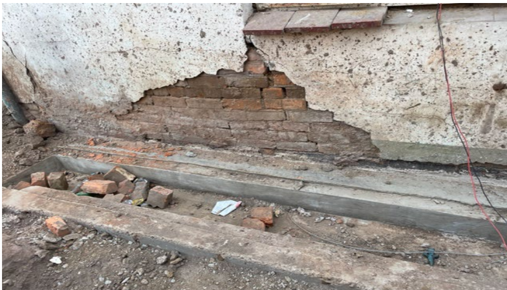
Picture showing the conditions of the walls of the buildings to be demolished
