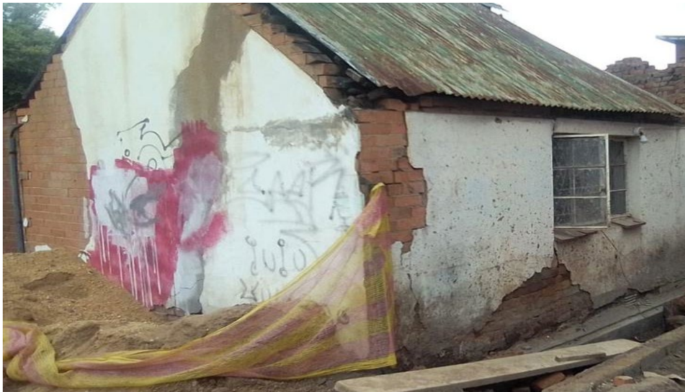
Picture showing the conditions of the roof for the building to be demolished
