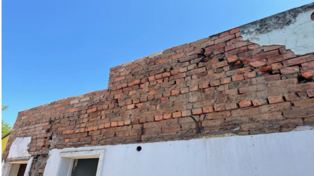
Picture showing the conditions of the beam filling for the building to be demolished
