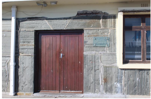
Lintels to be repaired & woodwork revarnished.
