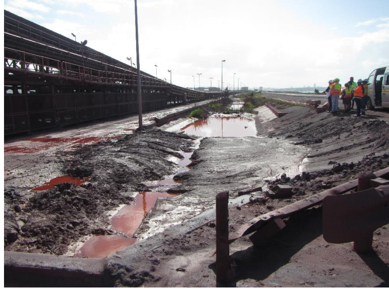
Sludge (contaminated water with iron ore) fill water channel.
