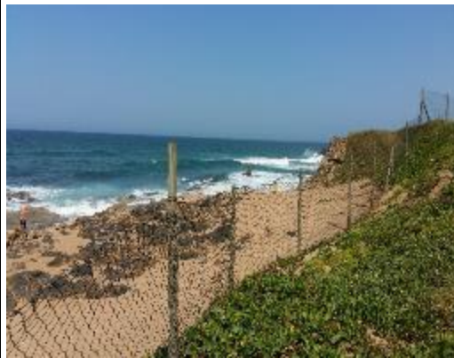
Figure 5 Southern view of sea wall location where wall is to be re-built
