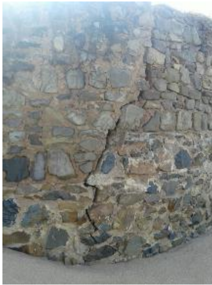
Figure 9 Evidence of fractures within remaining portion of sea wall.
