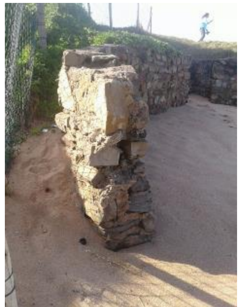
Figure 12 Section of wall requiring reinforcement of remaining portion and tie in to section to be rebuilt.
