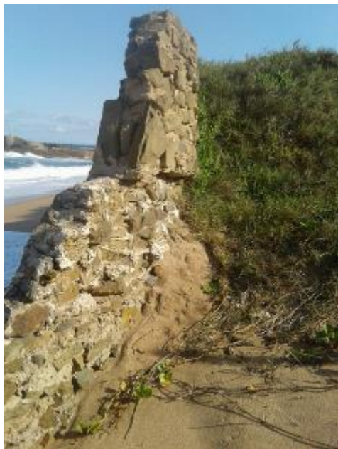
Figure 11 Section of wall requiring reinforcement of remaining portion and tie in to section to be rebuilt.
