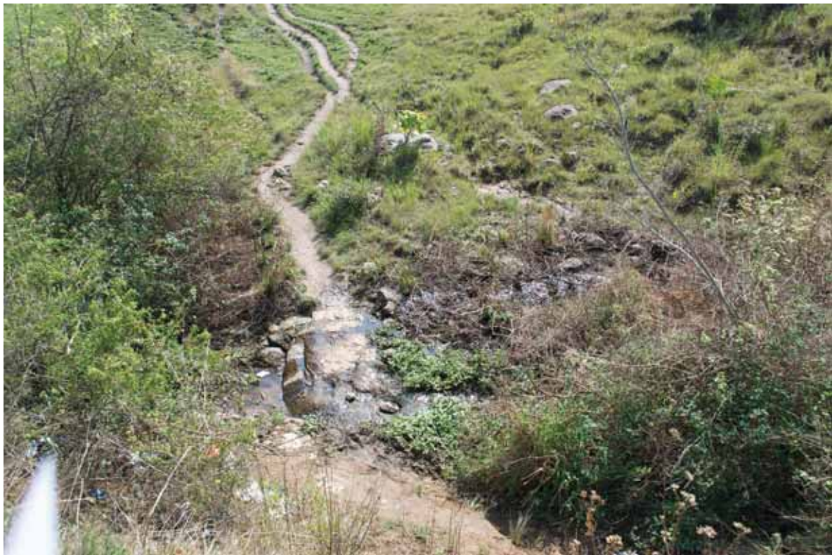
Plate 4. View of the site of the location of the culvert showing the reduced woody fringe and path devoid of herbaceous vegetation
