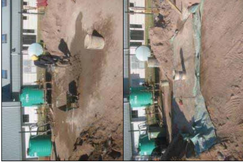
Figure 6: An example of mixing and moving concrete using an impermeable plastic sheet.
