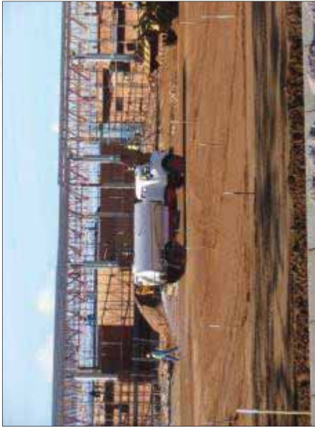
Figure 18: An example of dust suppression at a construction site to control dust generation.
