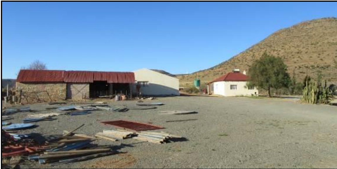
Photograph 3.12: Guest accommodation on The Dairy, with extensions in progress. A Noupoot WEF turbine is just visible between the buildings
