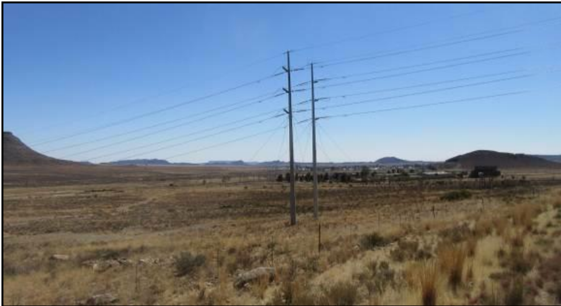
Photograph 3.43: Existing feed in Tx line from the Noupoort WEF which traverses the N9 between Barredeel rail siding and Midlandia.
