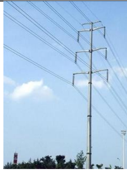
Plate 6-1: Concrete, steel or wood monopoles.
