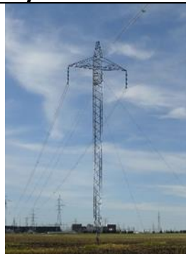
Plate 6-3: Free standing metal lattice towers.
