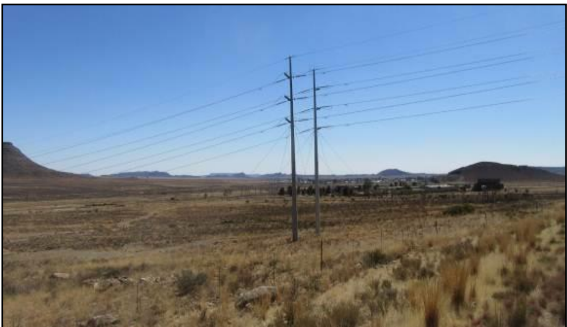
Photograph 7.20: Existing feed in Tx line from the Noupoort WEF which traverses the N9 between Barredeel rail siding and Midlandia.
