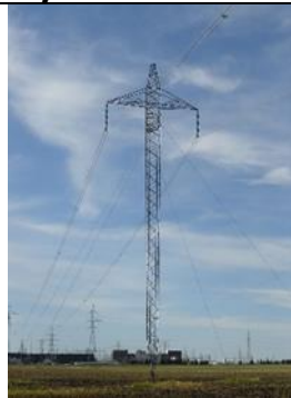
Plate 6-3: Free standing metal lattice towers.
