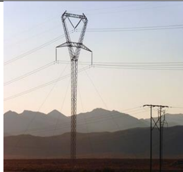
Plate 6-2: Guy line supported steel structures.
