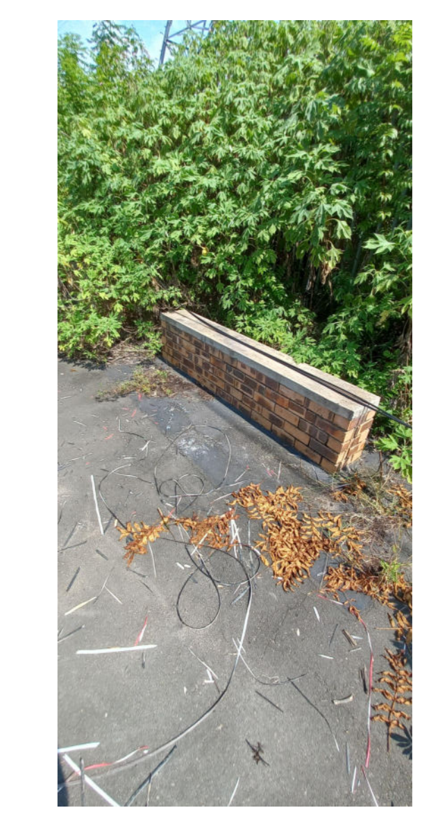
1. EXISTING PUBLIC SEATING (UNLAWFUL WORK)
