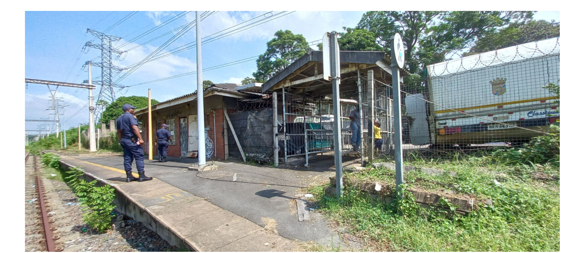
2. EXISTING ENTRANCE STRUCTURE (UNLAWFUL WORK)
