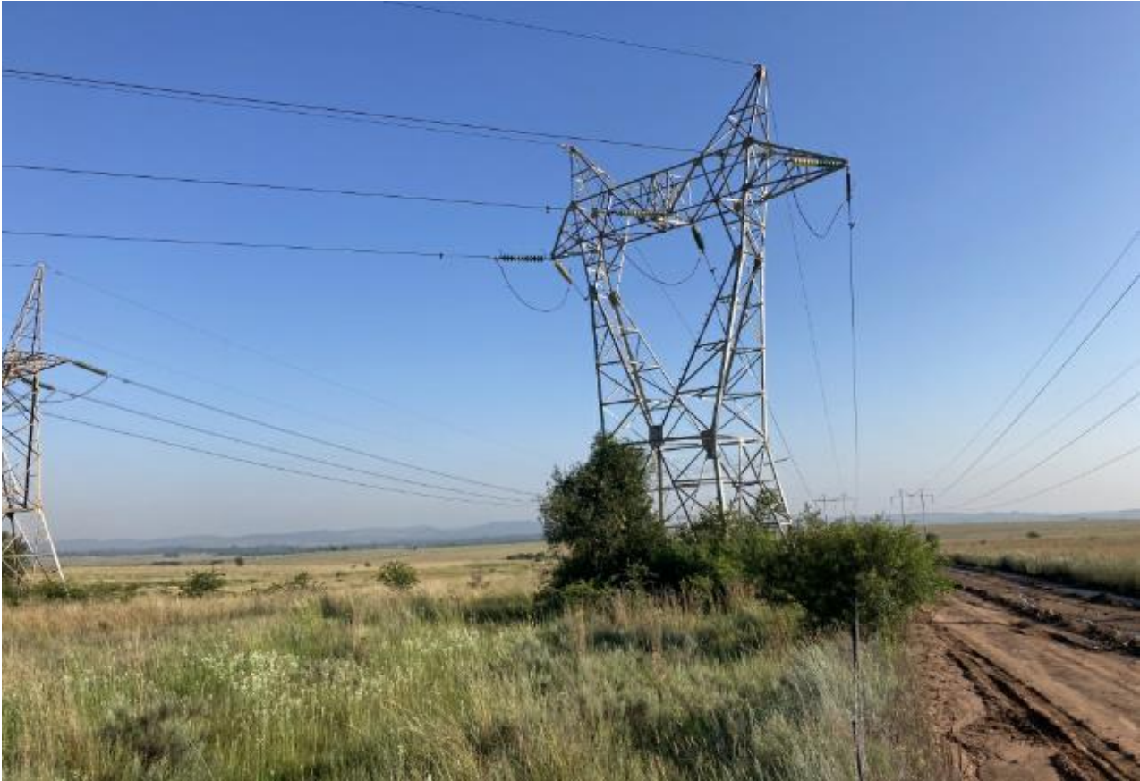
Figure 8: High voltage lines
