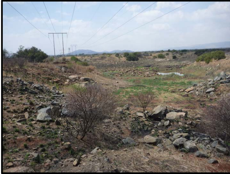
Figure 16 Excavation of soil and rock have taken place in the north western section of the study area
