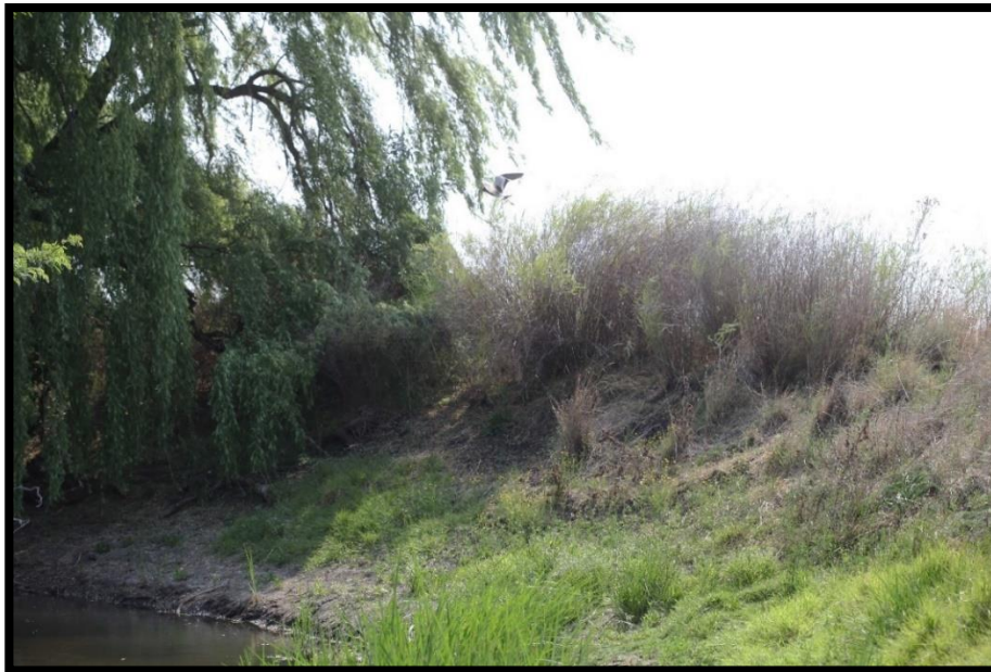
Photo 9 Walls of the active channel, the latter which cuts steep in the flat landscape, at the site. Photo: R.F. Terblanche
