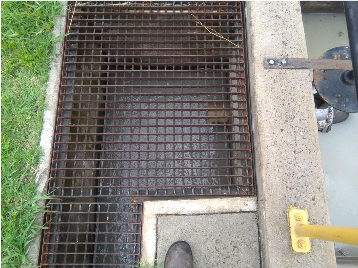
Figure 7-2 Oil separator system on the western border of the toll blending plant
