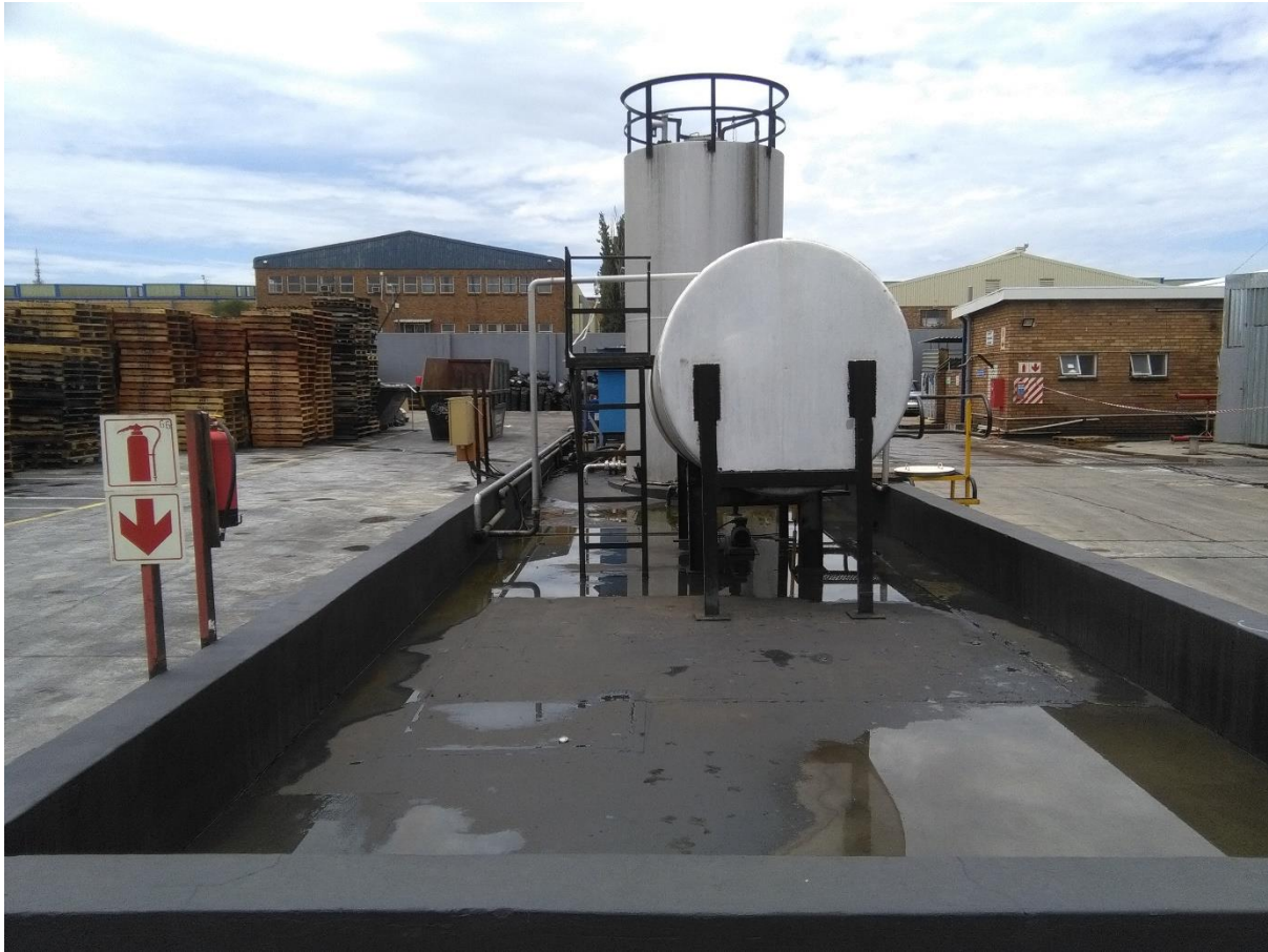
Figure 7-3 Example of a bunded wall that surrounds all storage tanks and hazardous waste at the toll blending plant
