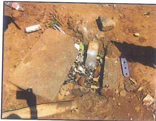
Plate 7-1: Blockages in drainage
