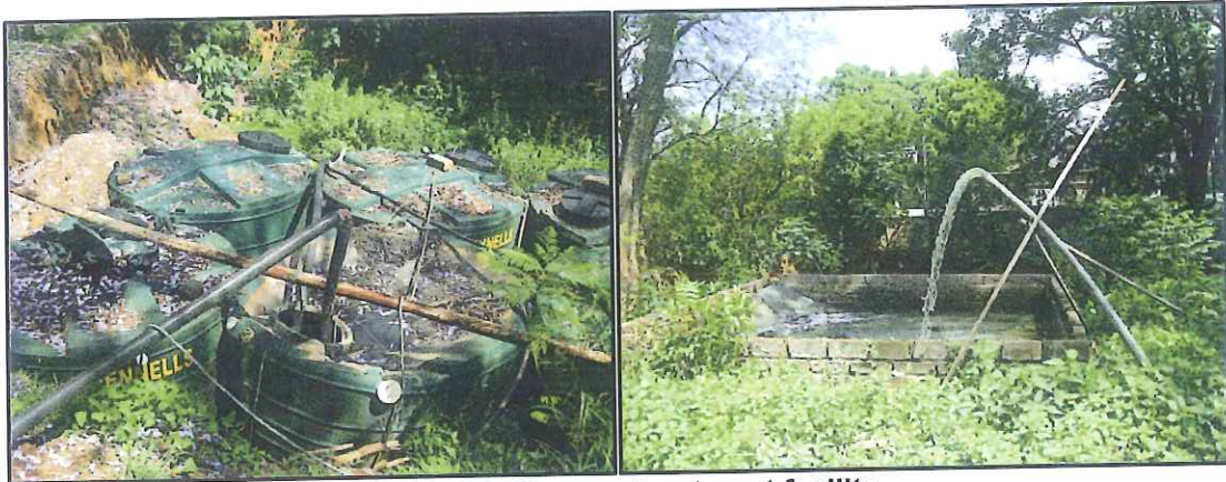
Plate 2-3: Sewage treatment facility
