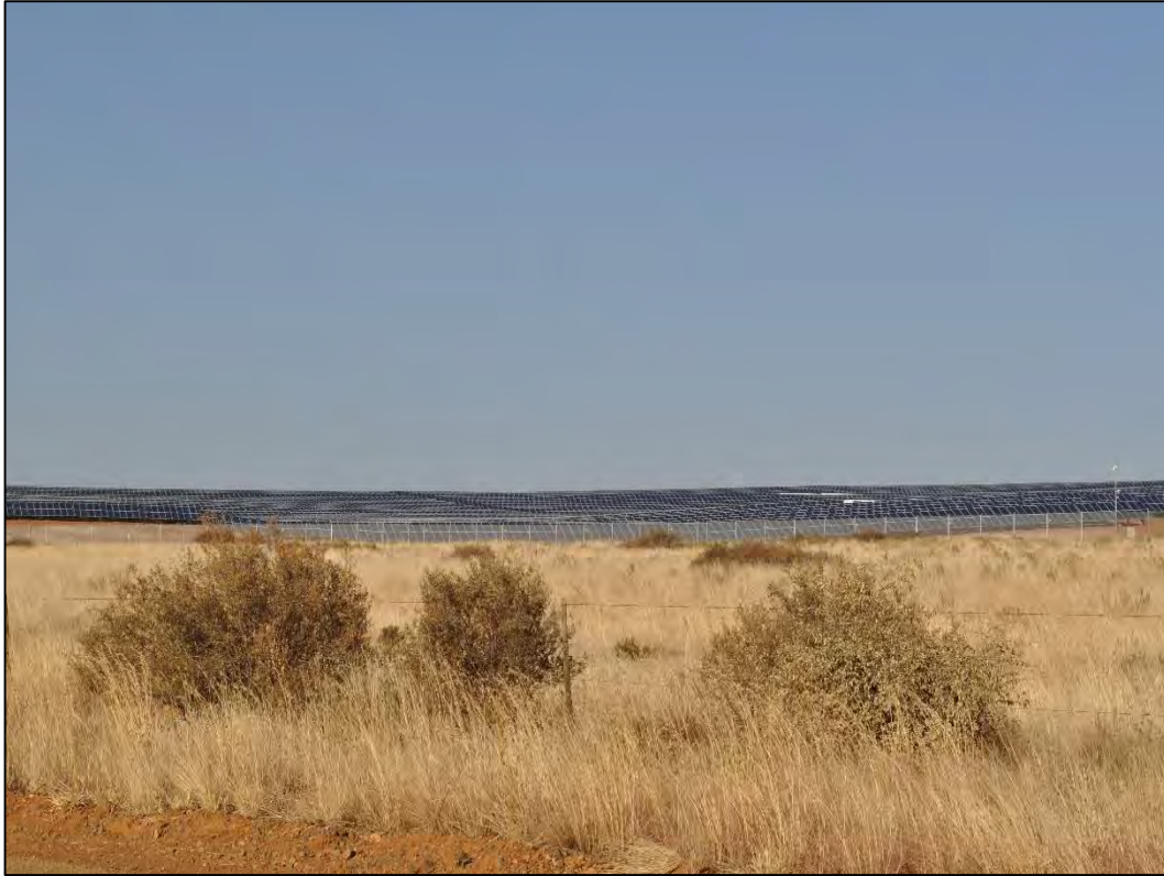
Figure 21: Photovoltaic Panels being erected near Lime Acres in the Northern Cape Province
