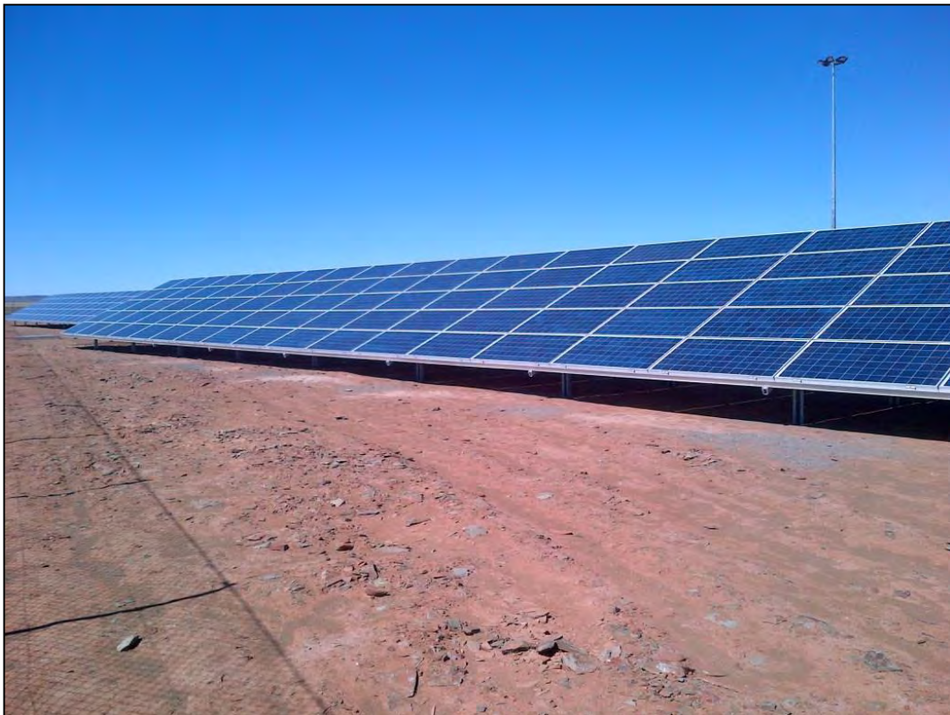
Figure 20: Photovoltaic Panels being erected near De Aar in the Northern Cape Province
