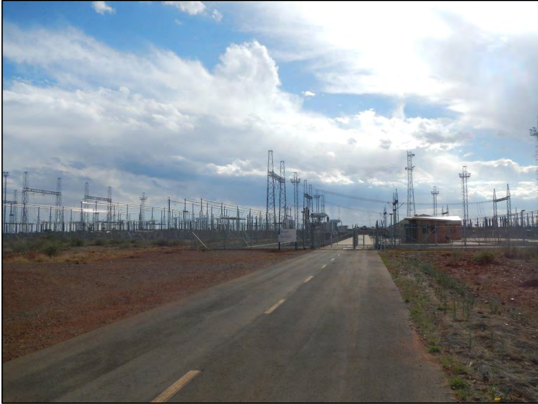
Figure 13: Eskom's newly constructed Mookodi Main Transmission Substation (MTS) which is located to the north-east of the application site, on the boundary of the visual assessment zone.
