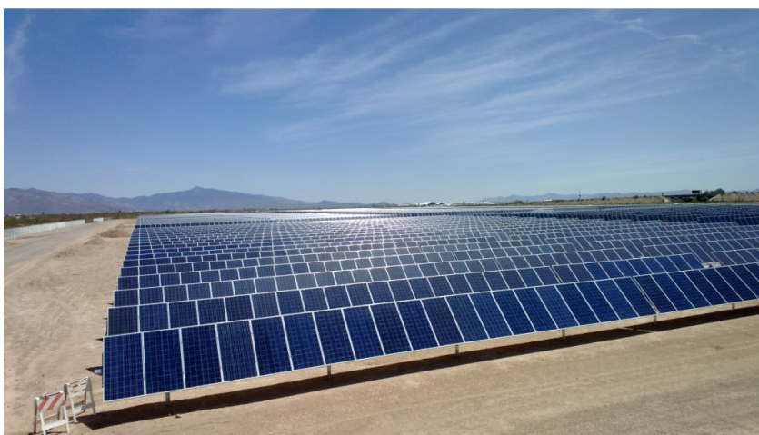
Figure 4: Illustration of tracking PV technology panels
