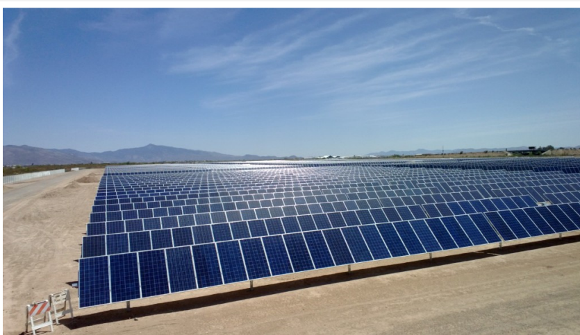
Figure 4: Illustration of tracking PV technology panels
