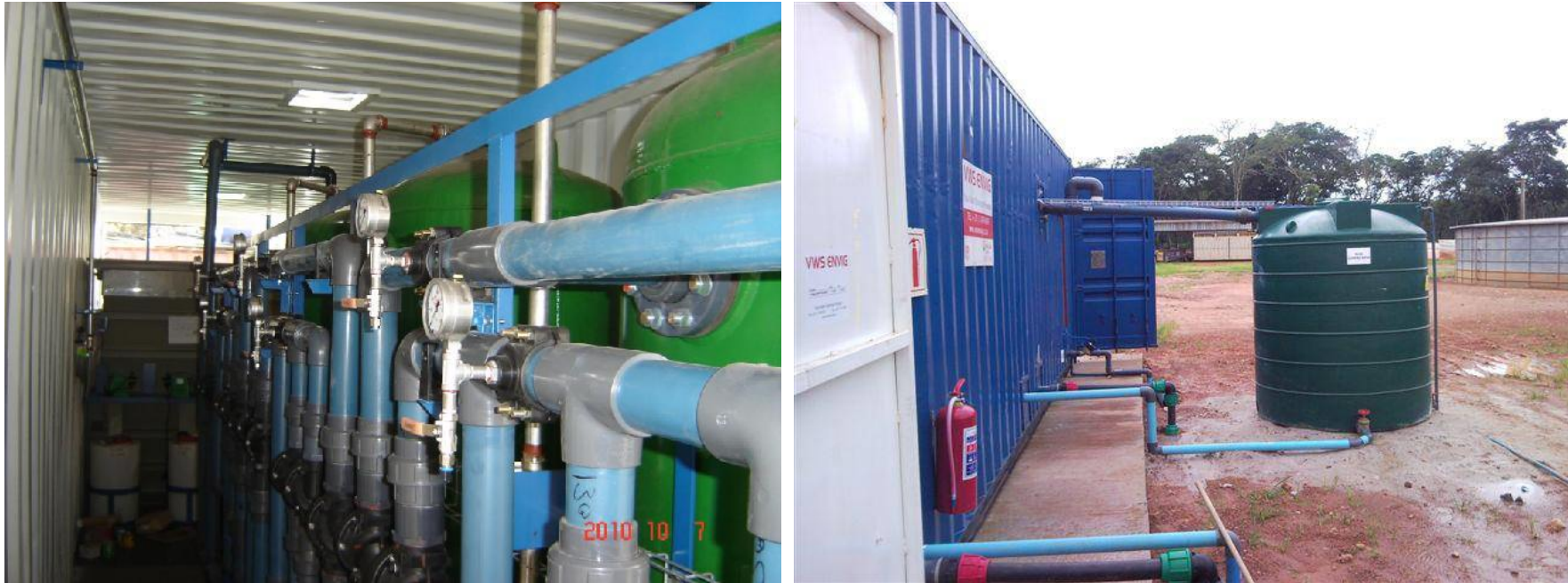
18 m 3 /h Lumwana Mining Co – Containerized water treatment plant – Zambia
