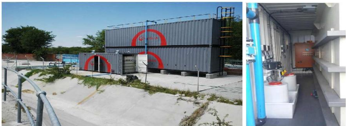
Figure 3: 180 m 3 /day Containerized STP - Letsholathebe Hospital, Botswana (31481536)
