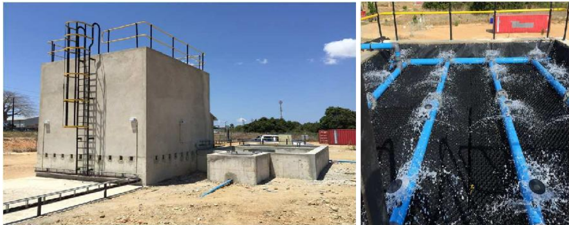
Figure 2: 100 m 3 /day Civil Based STP - Vale, Mozambique (31481539)
