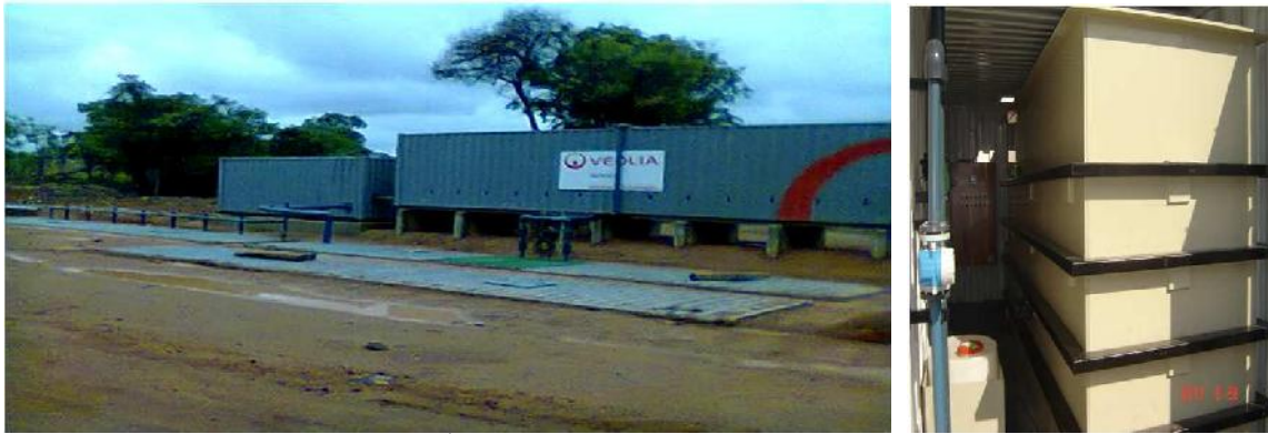
Figure 4: 110 m 3 /day Containerised STP - Kinsenda Copper, Congo (31481521)
