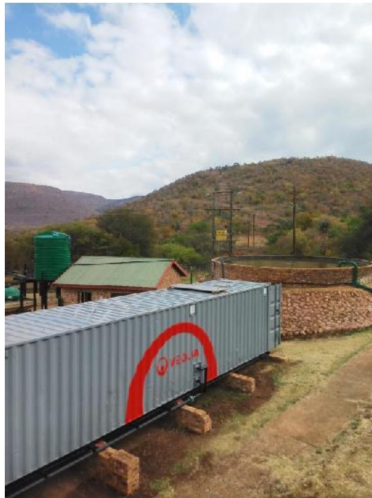
Figure 1: Typical Containerised Potable Water Treatment Plant
