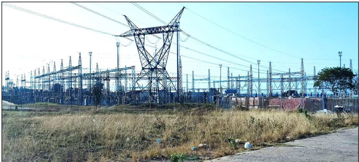
Images 3: The Acornhoek 275/132/22kV MTS Substation
