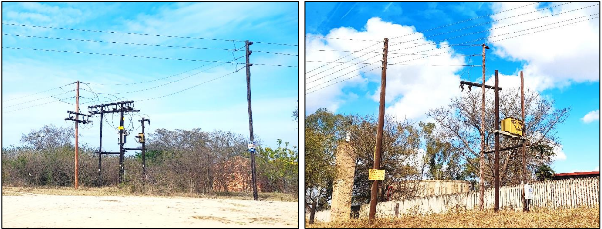
Images 4: The Site, Typical Overhead Medium Voltage (22kV) Lines
