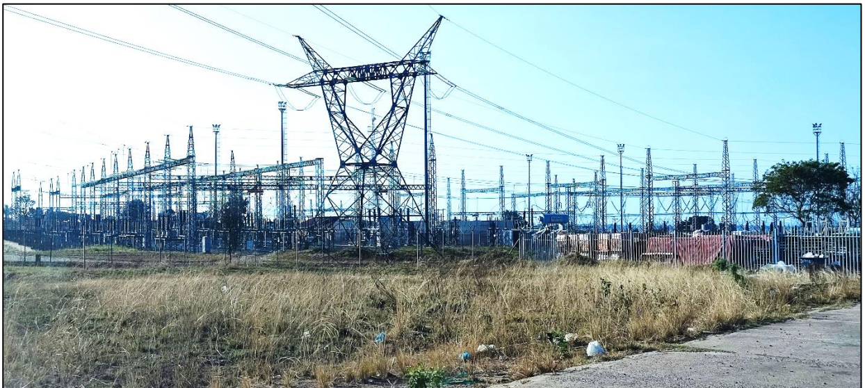
Images 3: The Acornhoek 275/132/22kV MTS Substation
