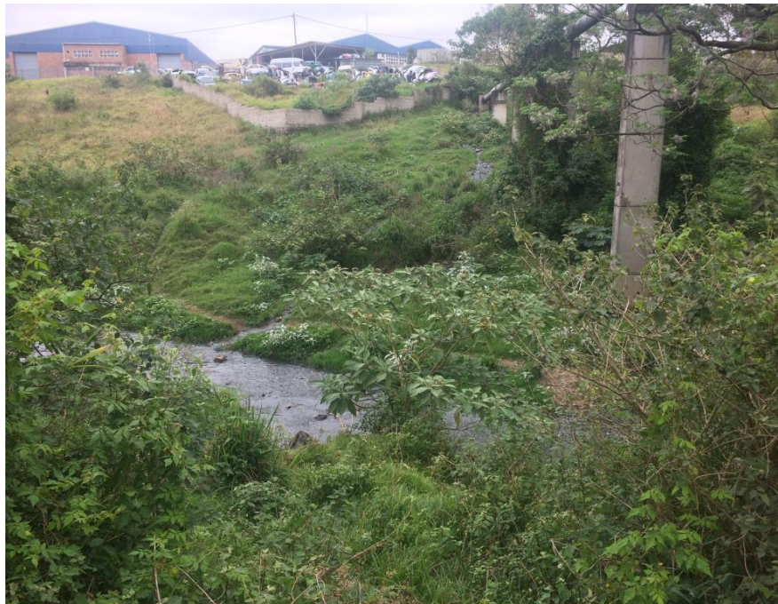
Figure 21: Sewerline across the tributary of the Mbozamo River (refer to top right of the image for the pipe and supporting columns)
