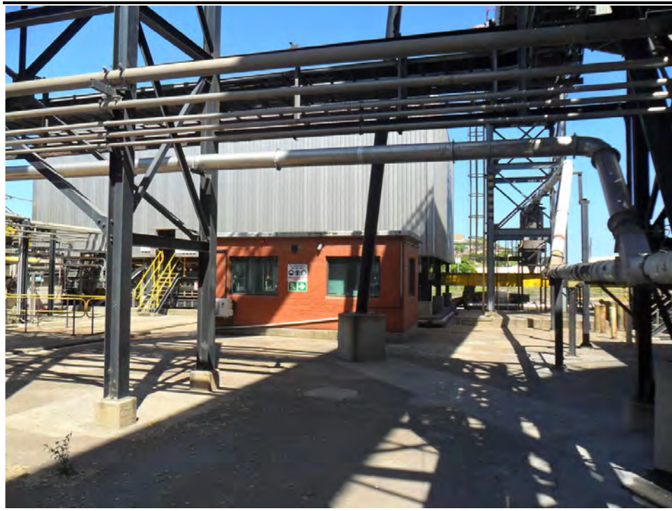
Figure 1.4 View from the HFO tanks facing east
