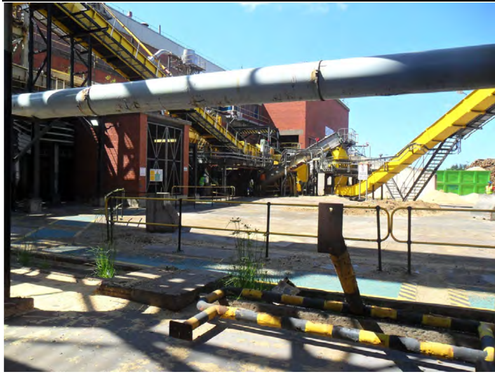
Figure 1.2 View from the HFO tanks facing north
