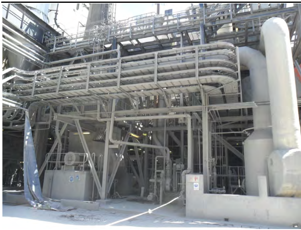
Figure 1.3 View from the HFO tanks facing south
