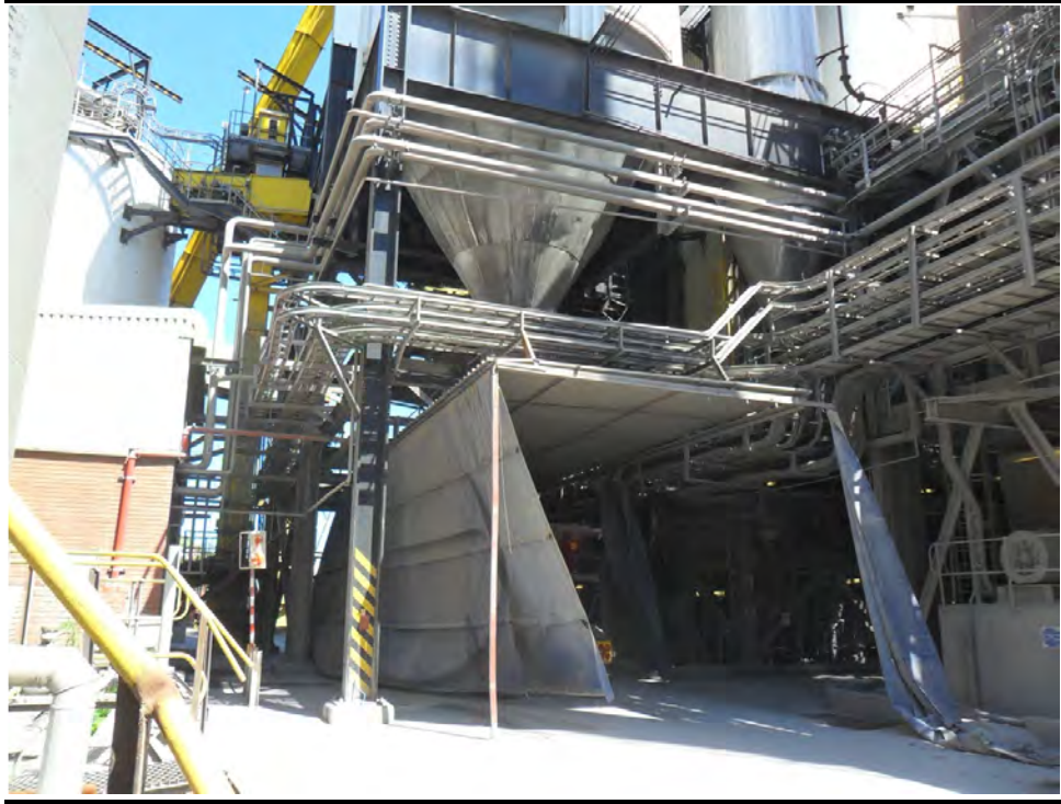
Figure 1.8 View from the HFO tanks facing south-east
