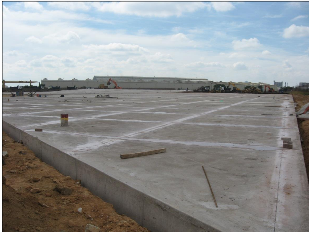
Figure 9: View of ongoing construction at the northern extent of the proposed site
