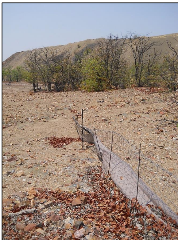
Figure 10. Flood damaged silt trap to be moved to the right into the tree line.
