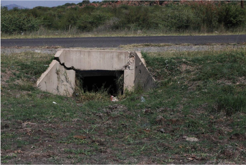
Photo 6 Culvert at the northern side of the tar road at Stream Crossing A. Photo: R.F. Terblanche
