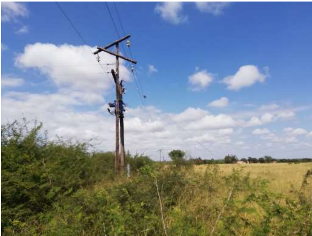
Figure 2 Existing MV on site
