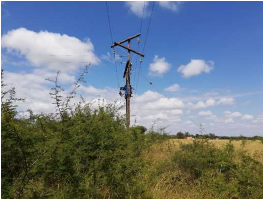
Figure 1 The t-off transformer position
