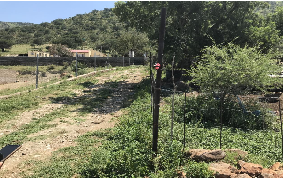
12. Picture no 12 : showing where the power line will be running and peg
