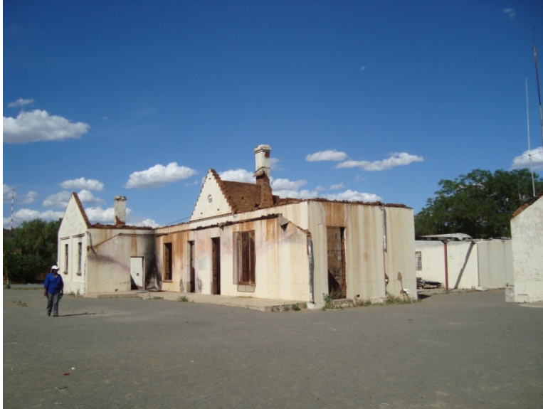
Figure 11. View of the town hall after burning down, view to north east.
