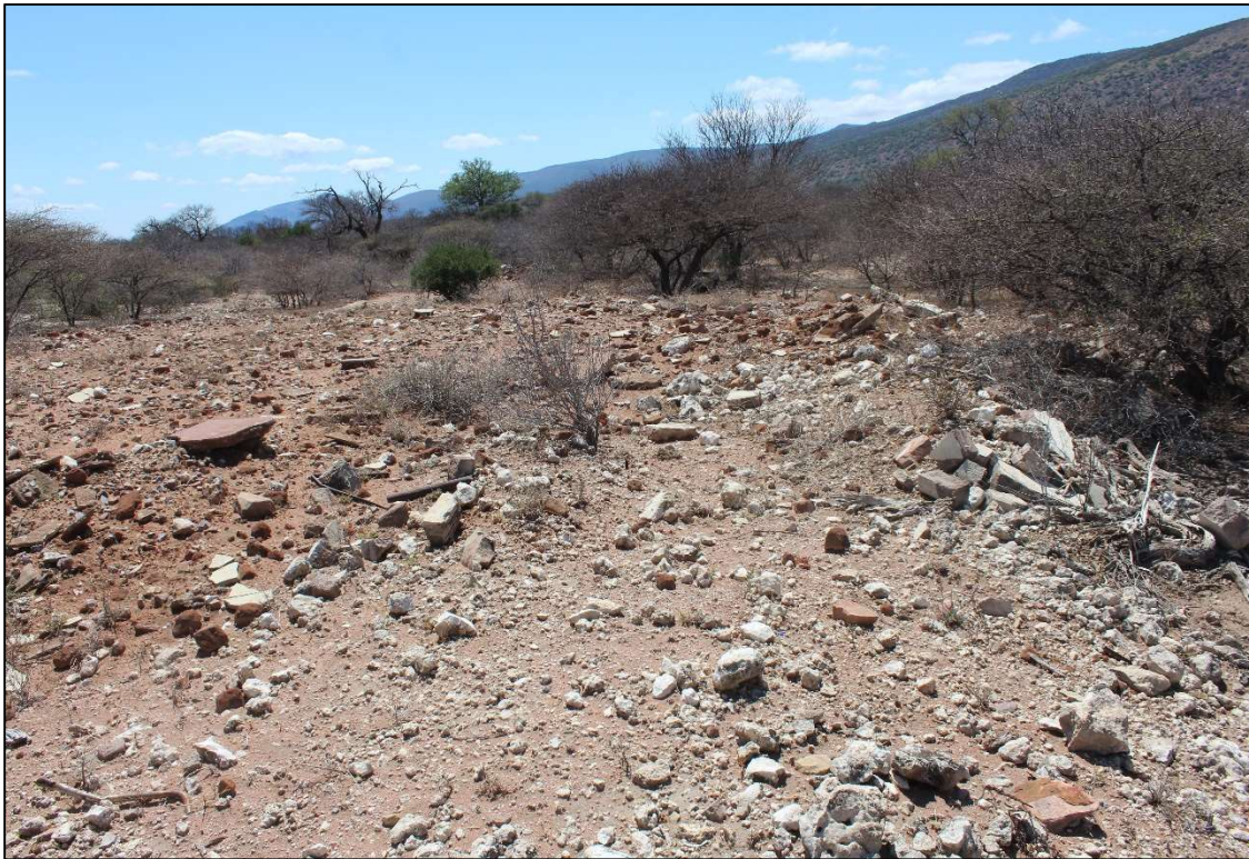
Figure 12: Rubble comprised of a mix of burnt clay bricks and concrete rubble
