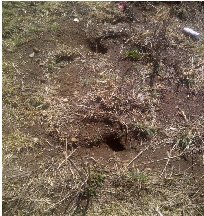
Figure 15. Holes observed during the field survey
