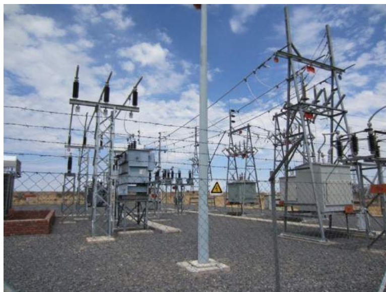
Figure 13: Schuitdrift Eskom substation
