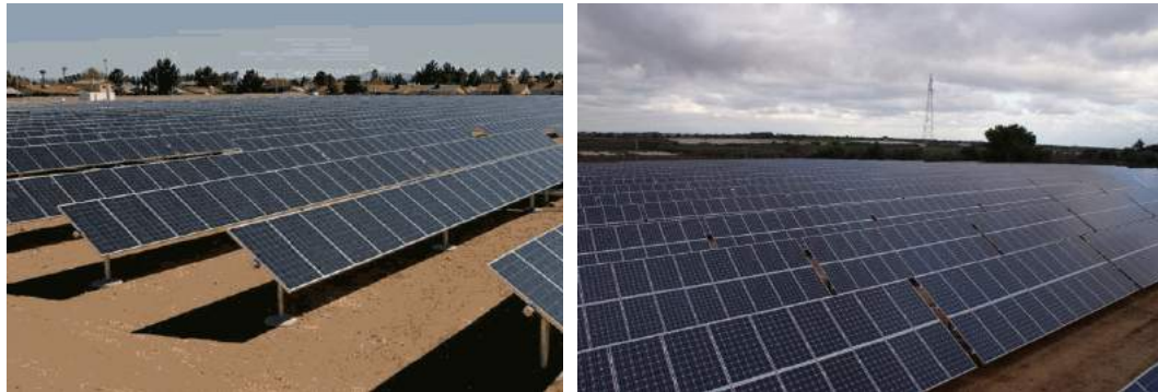
Figure 4: Typical layout of solar arrays
