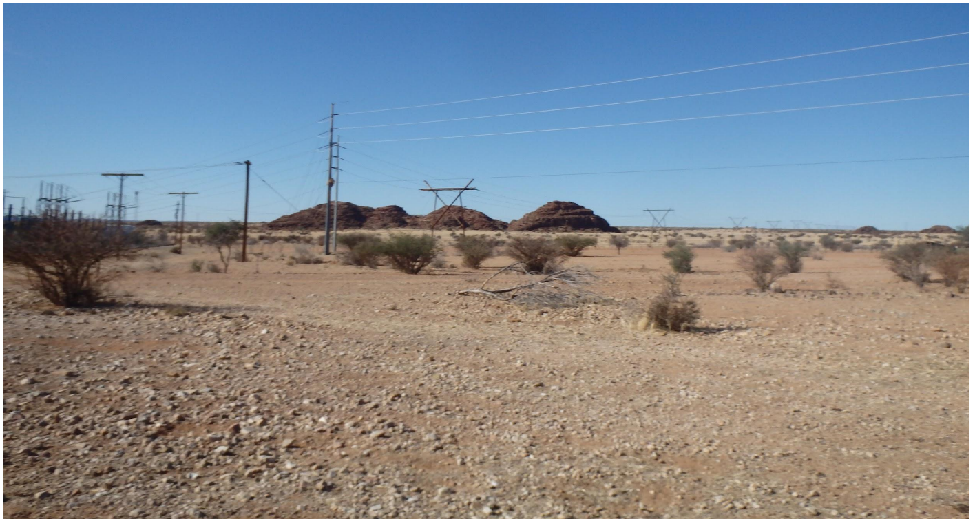
Figure 5.1 View of the substation near the Skuitdrift werf
